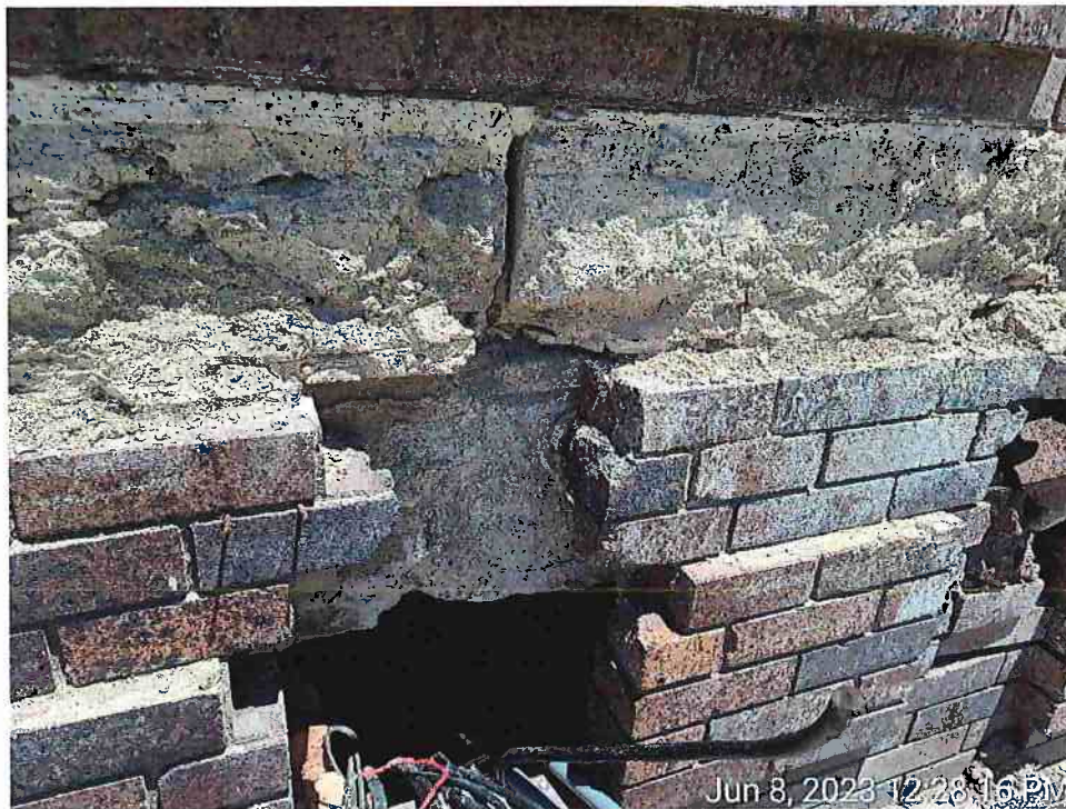
14. View of the removed brick on the exterior of the Building No Barrier Mastic Identified on the exposed Walls, Assuming Uniform Throughout
