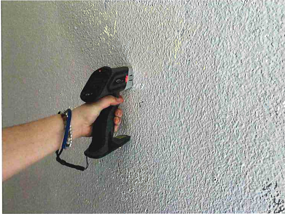
15. Typical view of the white plaster wall being tested for Lead-Based Paint
