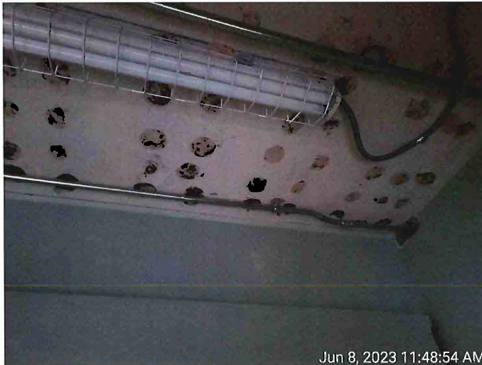
8. View of the exposed brown hockey pucks on the ceiling in the 3 rd Floor Closet negative for asbestos.
