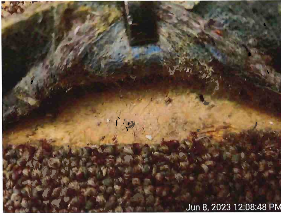
9. View of wood decking identified underneath the carpet in the Court House
