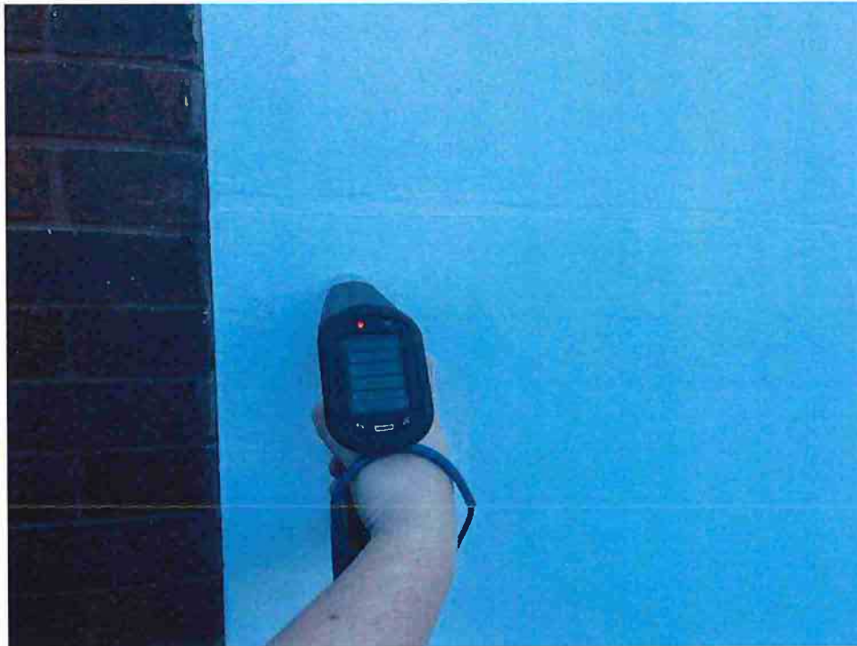
20. Typical view of the white exterior building components tested for Lead-Based Paint
