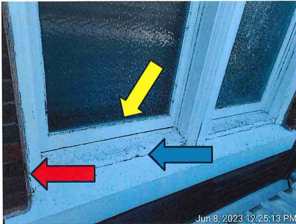
13. View of the samples collected. Red arrow indicates Red Exterior Brick Mold Caulking. Blue arrow indicates Exterior Window Frame Caulking. Yellow arrow indicates Exterior Window Caulking.
