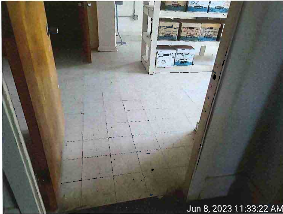
7. View of the asbestos-containing 9 x 9 inch White Vinyl Floor Tile adhered with Black Mastic identified in the Records Room on the 3 rd Floor
